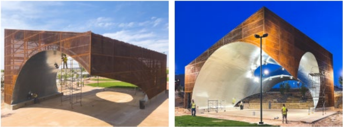
Rio Rancho Campus Park | Under Construction Six-Acre Park with Sky Room Performance Pavilion & Amphitheater $3,200,000
